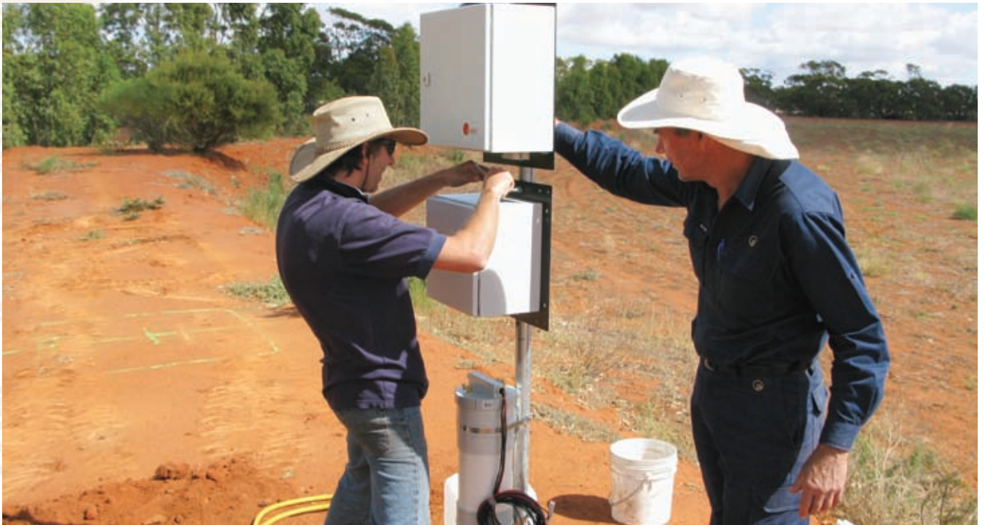
DAFWA Technical Officers James Newman (left) and Kevin Denham install a TELS unit in Perenjori similar to those planned for SWCC towns.
