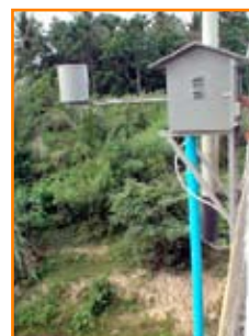
An installed rain gauge in Thailand.
